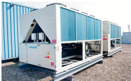
Chillers Chillers are used for cooling large commercial spaces and are often found in office buildings and industrial settings.
