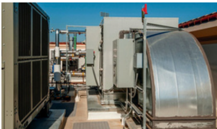
Centralized Commercial HVAC Systems (These are large-scale systems designed to cool entire commercial buildings. They include rooftop units, chillers, and air handling units.)
