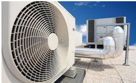
VRF (Variable Refrigerant Flow) Systems VRF systems provide efficient heating and cooling for larger commercial spaces. They offer zoning capabilities and can simultaneously heat and cool different areas.
